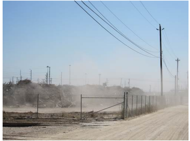
Excessive Dust Issues
